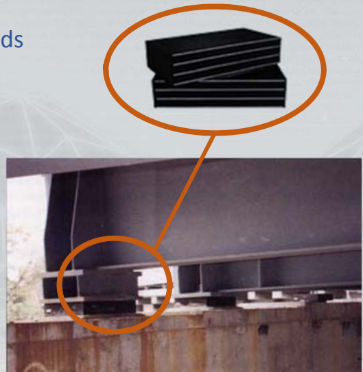
Building support steel on 6.5Hz rubber bearing pads
