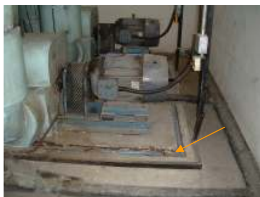
Pump installation with “Sylomer®” in replacement to the original Cork pad (for reducing vibration transmission to structure)
