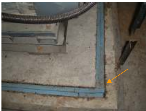
Close-up showing exposed 2 layers 25mm Sylomer® R pad edge at concrete plinth
